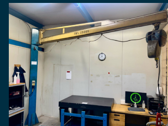
Lot 229: UNKNOWN MFR 250Kg SWL Jib Crane with Electric Hoist
